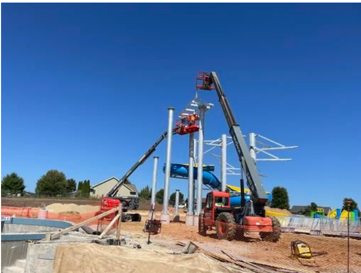
Start of installation of Waterslide. Added on Sep 15, 2023, 10:56 AM CDT Added by andrew gordon
