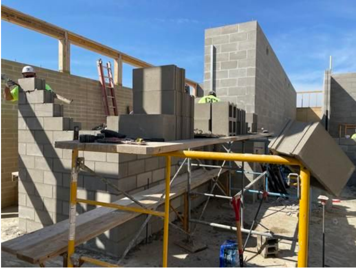
Installation of CMU on interior of Bath House Added on Sep 15, 2023, 11:50 AM CDT Added by andrew gordon
