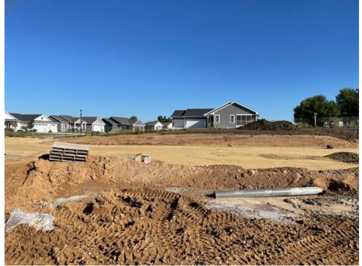
start of grading for north Parking Lot. Added on Sep 15, 2023, 10:59 AM CDT Added by andrew gordon
